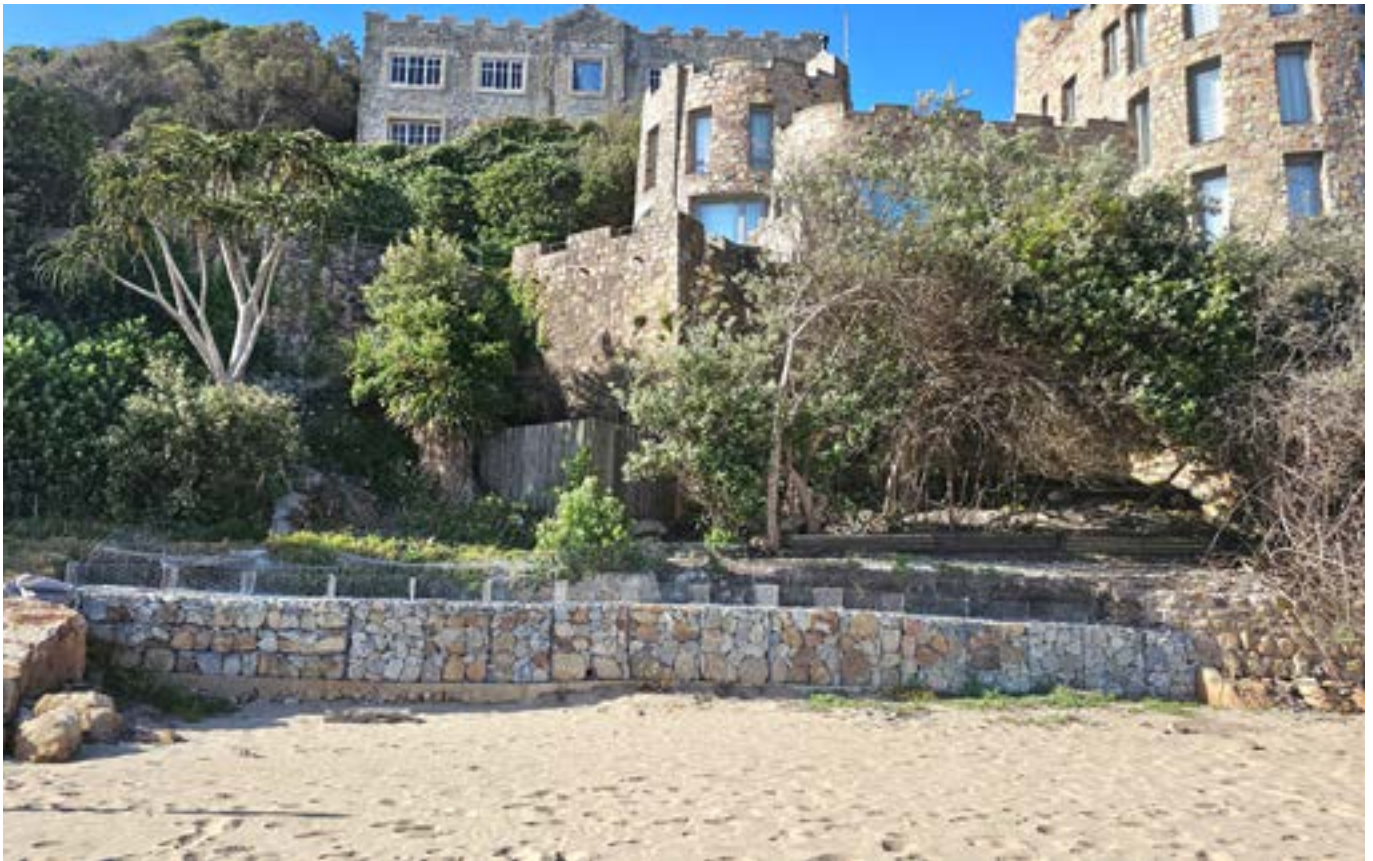
GABION PROTECTION: This gabion wall allows high seas to move through the gaps between the stones, reducing the force of the water. Stones are packed behind the gabions, giving another layer of protection to the footpath. This was paid for with national disaster funds, topped up by the Knysna Municipality.
