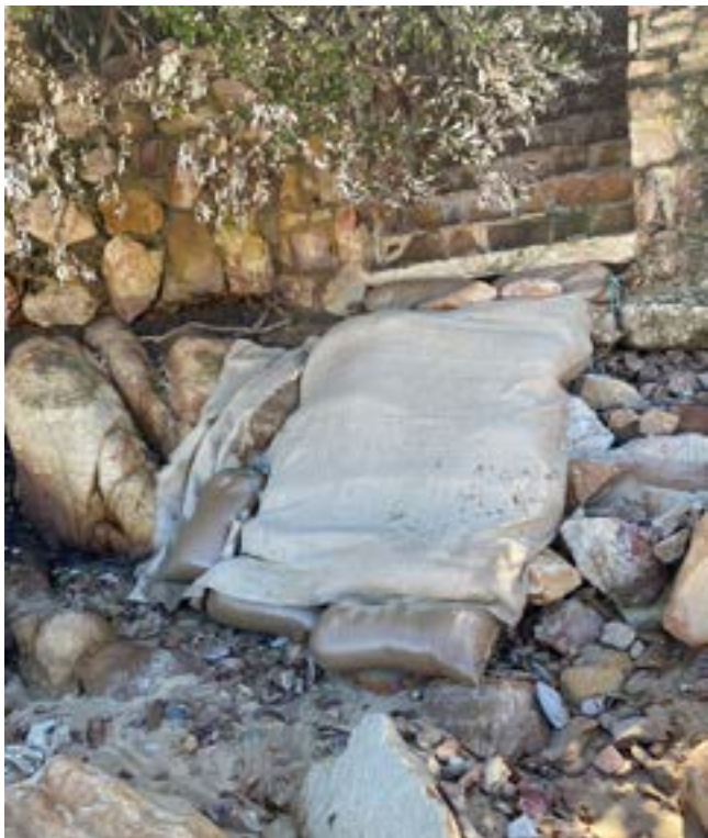
SANDBAGS: The 2023 storm surge swept away sand, leaving the steps from the footpath below Montrose about a metre above the beach.
