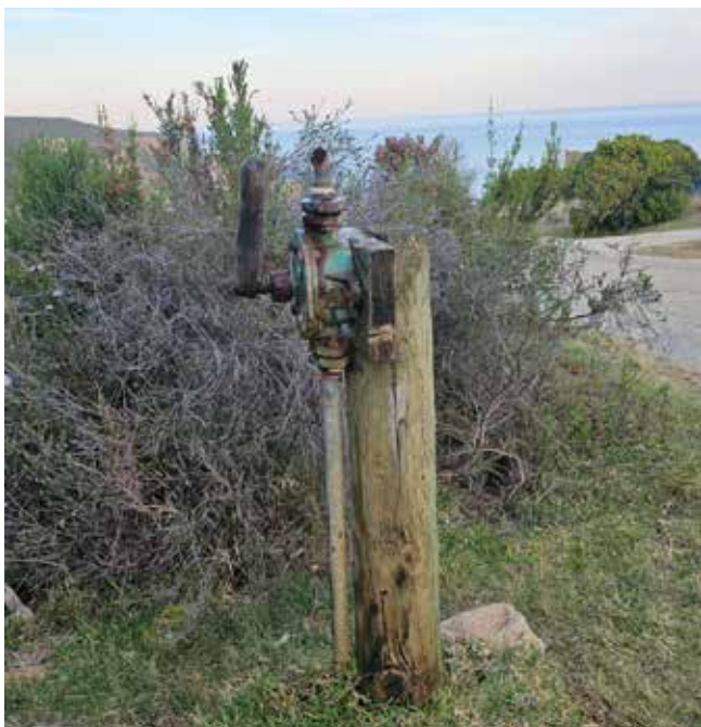
Sadly, someone stole the copper spout from the pump on the tank on the headland that Julie put there for the public. There is no drinking water at the beach, and this water is used daily mainly by fishermen and children who walk to Noetzie.
